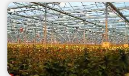
Greenhouse CHP and CO2 Dmitrov, Russia 5.4 MW | 3 x J612
