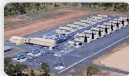
Coal mine gas Moranbah mine, Australia 45.6 MW | 15 x J620
