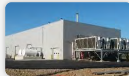
Diesel-to-Gas Switching Coldwater, MI, US 13MW | 3 x J624
