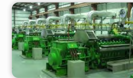
Rural electrification Bangladesh 81 MW | 28 x J620
