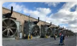
Gas Compression (high BTU field gas) Harrison Co, WV 7044GSI
